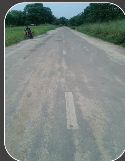
Jan 2020 – 6 years later with no maintenance. The road is 100%
